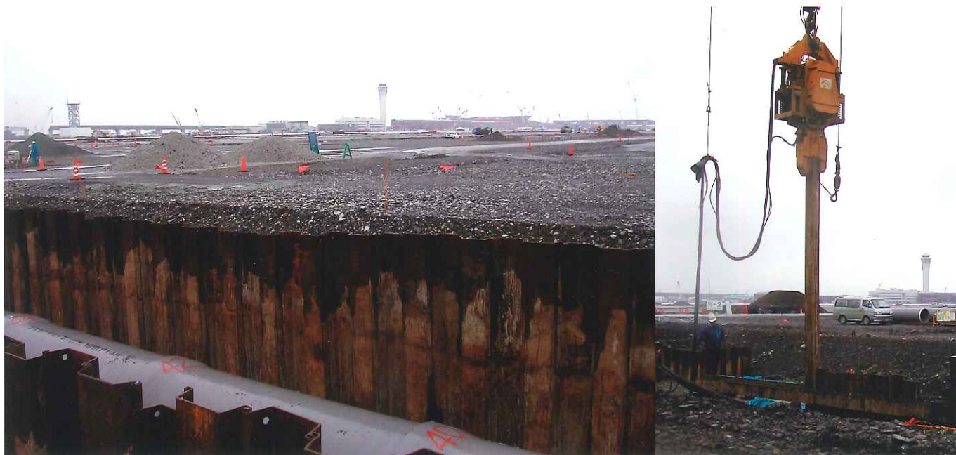
The Centrair airport rainwater drainage pipe institution construction. Orderer: Central Japan International Airport Co., Ltd. Construction company: Kumagai / Nishimatsu / Tokura JV
